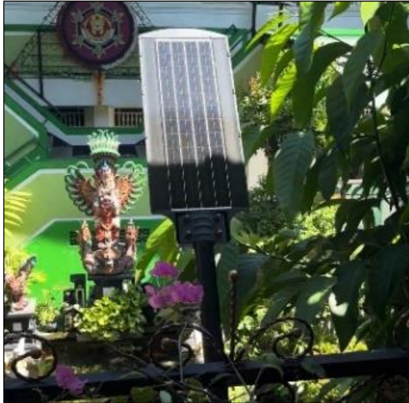
Figure 9. Solar Panel Placement
